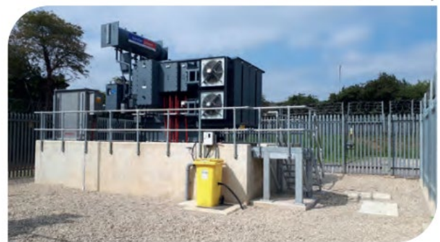
Elevated substation at Drakes Way
