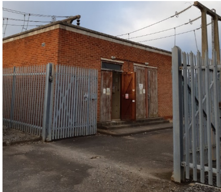
Figure 21 Example of 'typical' substation building – Headington Rd, Oxford.
