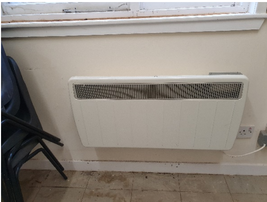
Figure 24 A typical electrically heated convector unit found in substation buildings.
